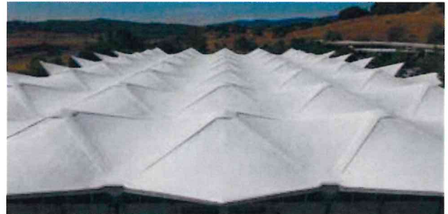
SPF roof installed over an unusual roof design at Birkenstock headquarters in Novato, CA.
