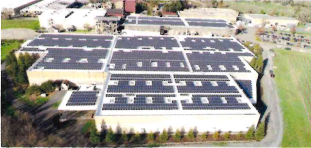
SPF roof with photovoltaic panels at the Rodney Strong Vineyards in Healdsburg, CA.
