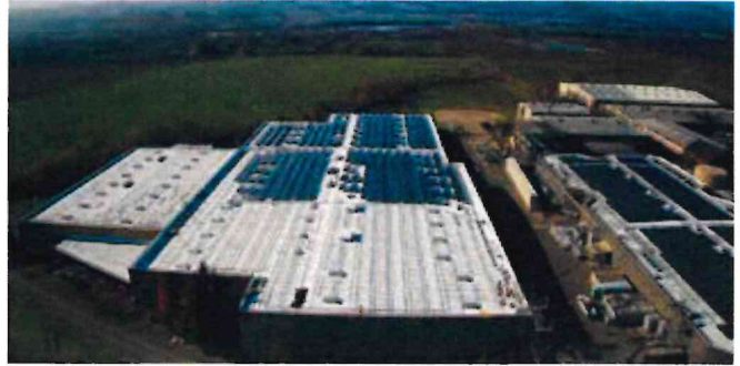
SPF Roofing installed below roof-mounted photovoltaic panels (during panel installation) on the Rodney Strong Vineyards facility, Healdsburg, CA.
