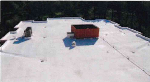
SPF roofing applied promotes enhanced drainage. IMAGE COURTESY OF CENTRAL COATINGS, MADERA, CA
