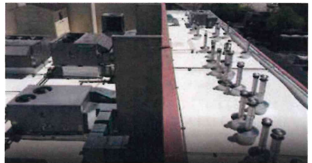
SPF provides self-flashing around all deck-mounted equipment and penetrations for this industrial manufacturing facility.
